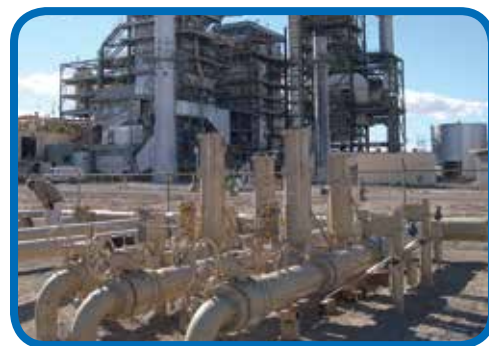
Figure 10 - Slam Shut and Fast-Acting Monitor Regulators Natural Gas Fired Power Plants (Power Generation Industry)
