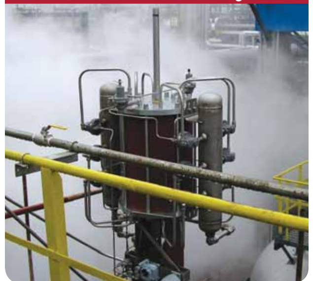
SVI II AP on steam conditioning valve
