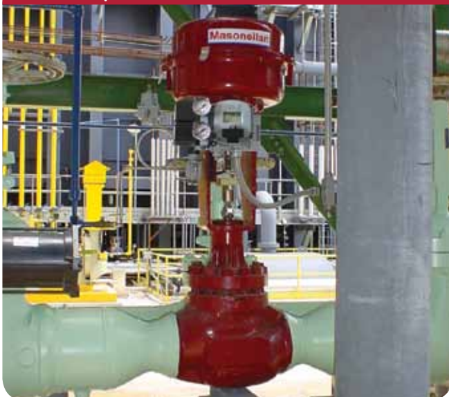
SVI II AP positioner on severe service valve
